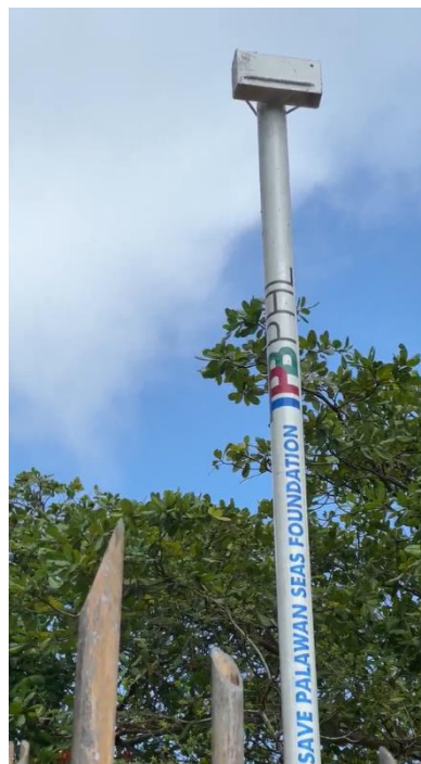
One of the solar light posts installed in Sitio Calabugtong
